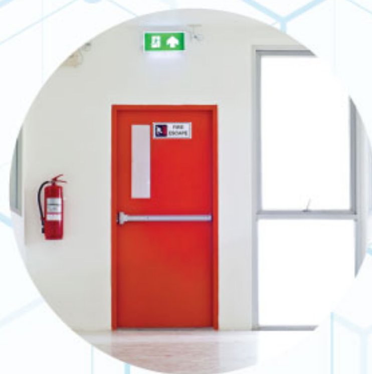
FIREDOOR / WINDOWS PERIMETER
