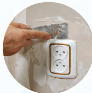
GAP AROUND POWER OUTLET
